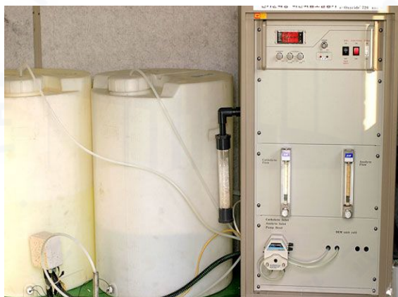
Figure 3.1 Photograph of ClO 2 generator
